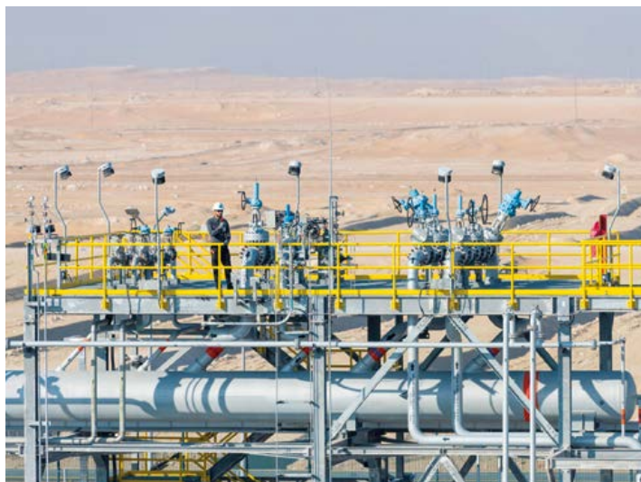
▲ Hawiyah Gas Compression Plant, Saudi Arabia
