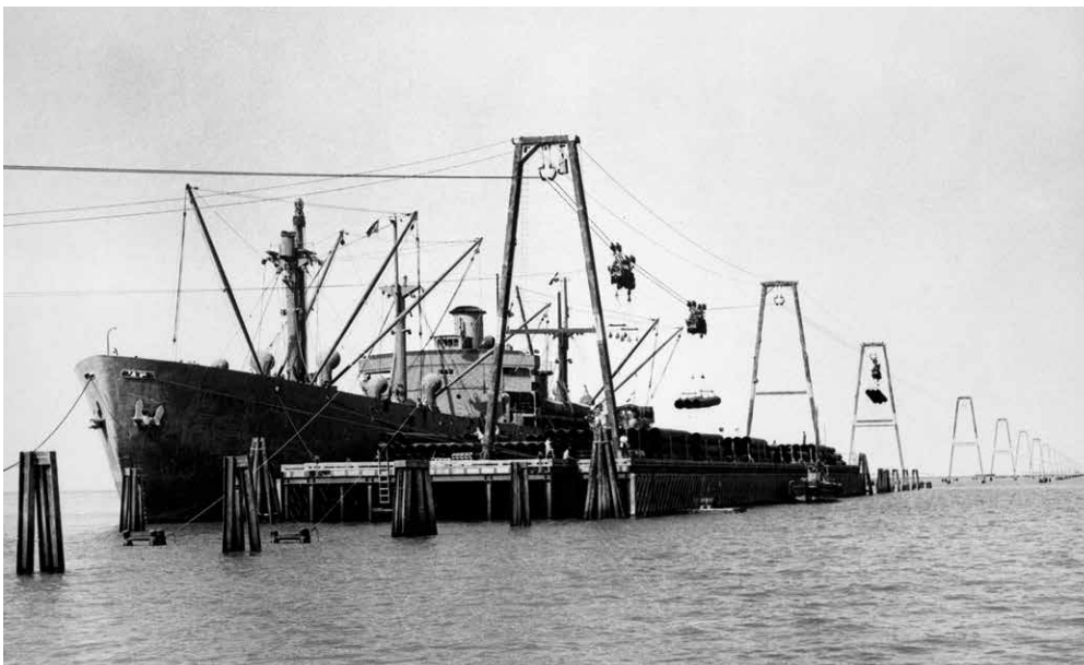
Sections of pipe are unloaded from a ship by the Sky Hook aerial tramway in 1948. Once ashore, the sections of pipe were welded together into longer lengths and sent into the desert on massive tractor trailers.
