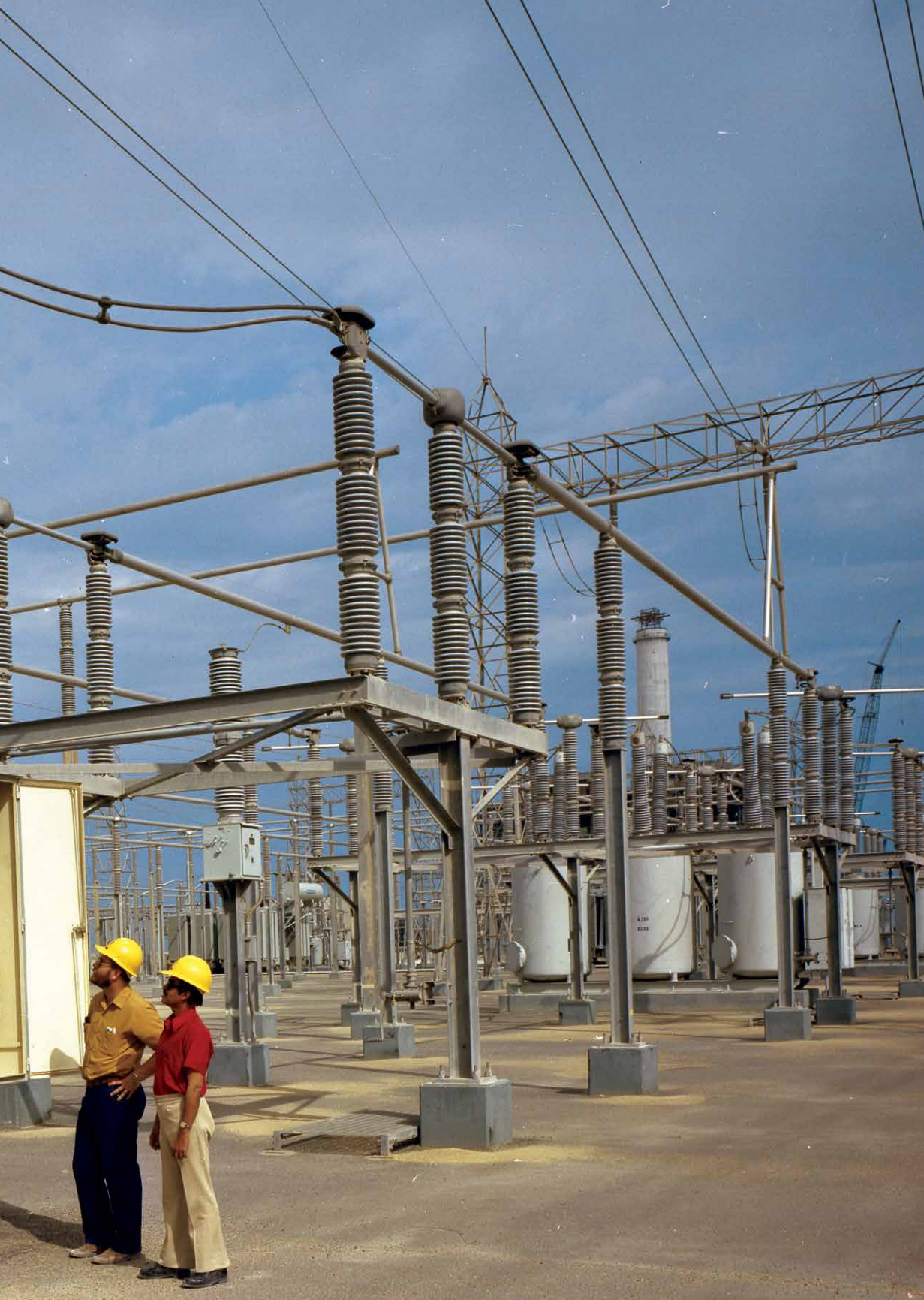
One of Aramco's most challenging projects in the 1970s was unrelated to oil: the creation of a unified electrical power grid in the Eastern Province. The facility in this 1979 photo, one of a pair located near Ju'aymah, began operations that year, increasing the total capacity of the Saudi Consolidated Electrical Company (SCECO) to almost 1,900 megawatts.
