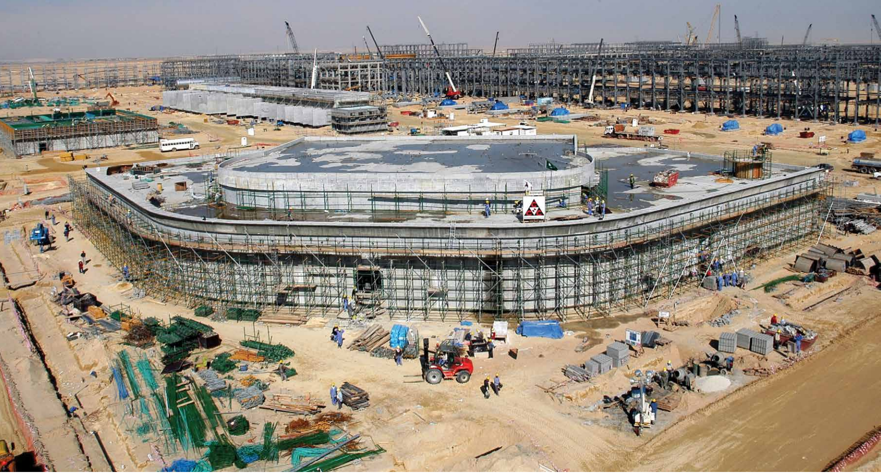
The massive Khursaniyah oil and gas-processing complex, shown here during construction, was built to process 500,000 bpd of Arabian Light crude oil and 1 billion scfd of associated gas.
