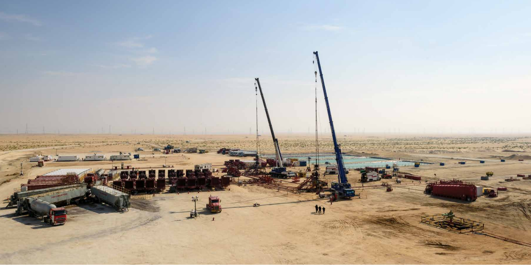
Cranes work in the Jafurah field — site of the largest unconventional gas field in the Kingdom.
