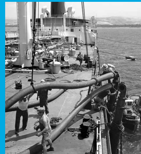
A combined crew of Tapline and oil tanker personnel hoist submarine crude oil loading lines aboard ship in July 1961, an action repeated thousands of times over the life of the Tapline terminal at Sidon, Lebanon.
