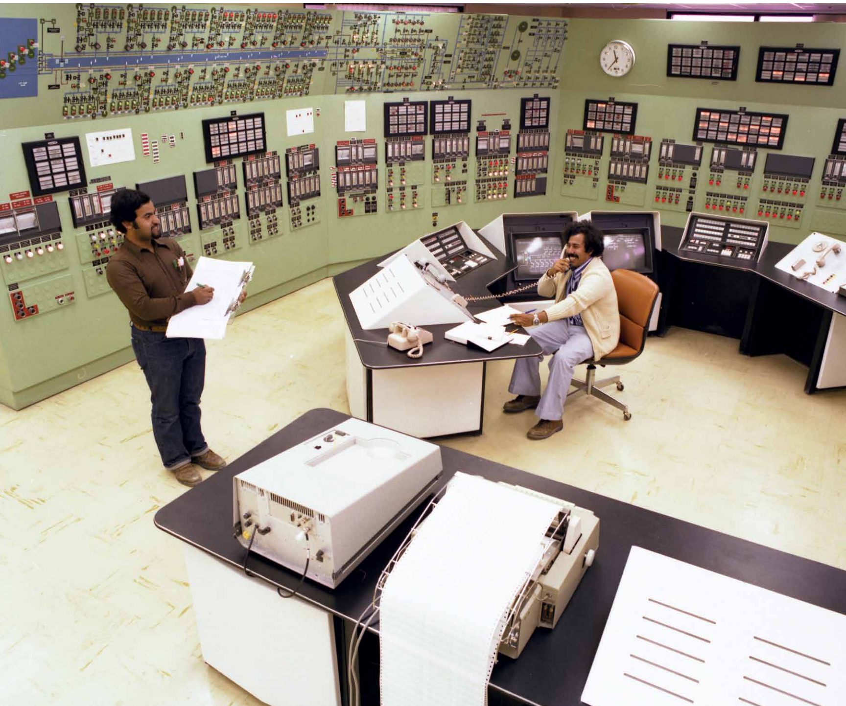
Operators in the control room of the Qurayyah Seawater Treatment Plant in 1979 monitor the processing and delivery of 4.2 million bpd of seawater for injection into oil fields to maintain reservoir pressure.
