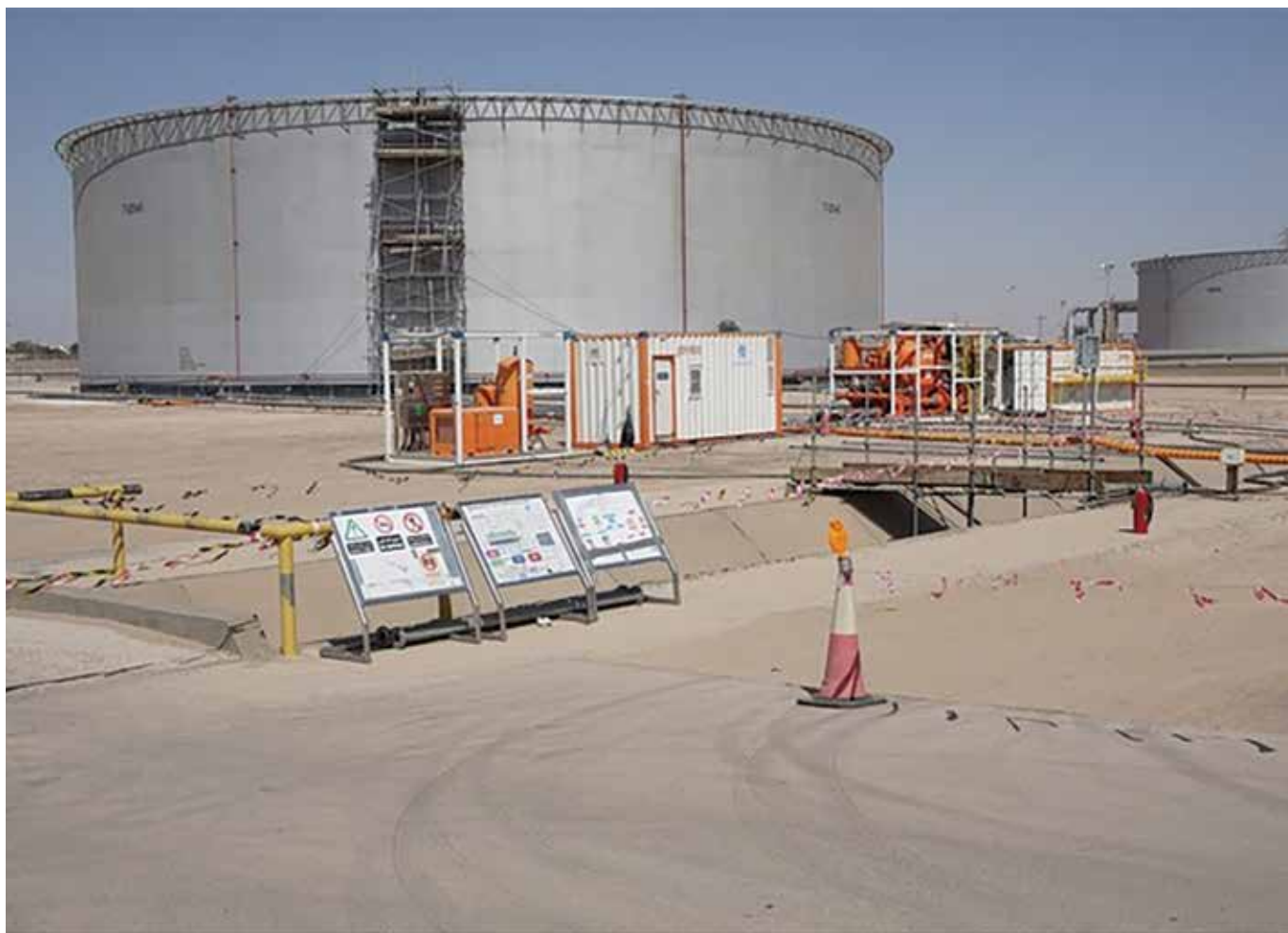
Figure 1. Overview of T-2041 and ATC custom equipment. (Photo Source: Saudi Aramco)
