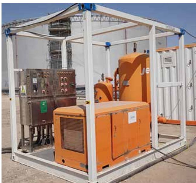
Figure 2. Air compressor Unit
